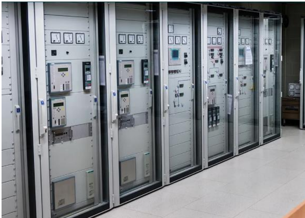
Figure 4 - Relay panels in a substation control rom. The panels contain different components related to the control system in a substation. The panels typically contain IEDs, measurement indicators, buttons, switches, RTU etc. [7].
