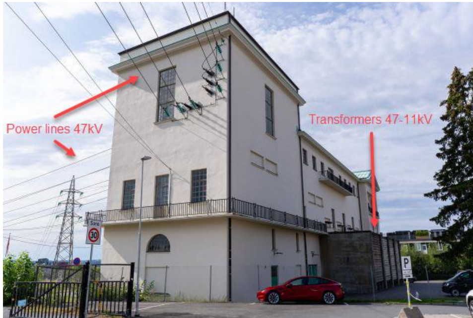
Figure 2.1 - Tonsen substation, located in Oslo and owned by Elvia. The figure shows high voltage lines (47kV) entering the building. The grey concrete cells in lower-right part of the figure house the transformers. The transformers transform the voltage to 11kV and deliver power through cables to the distribution network [3].
